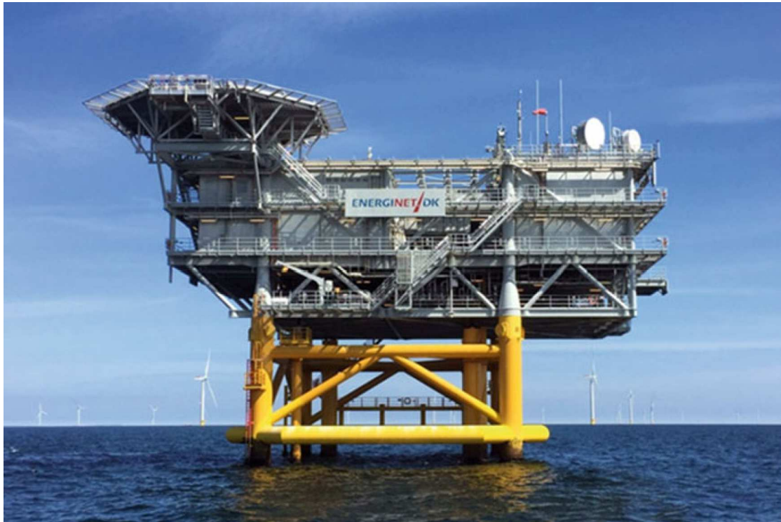
Fig. 2 The substation used for recording behavioural reaction of migrating raptors. The closest turbines are seen in the background (c. 1.8 km away)
